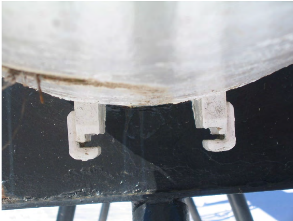
Photo 10: Rail Lug, Longitudinal View
